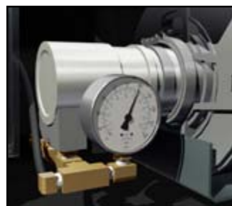
Figure 17. Black needle on pressure gauge showing PSI while system is in service or in flush mode.
